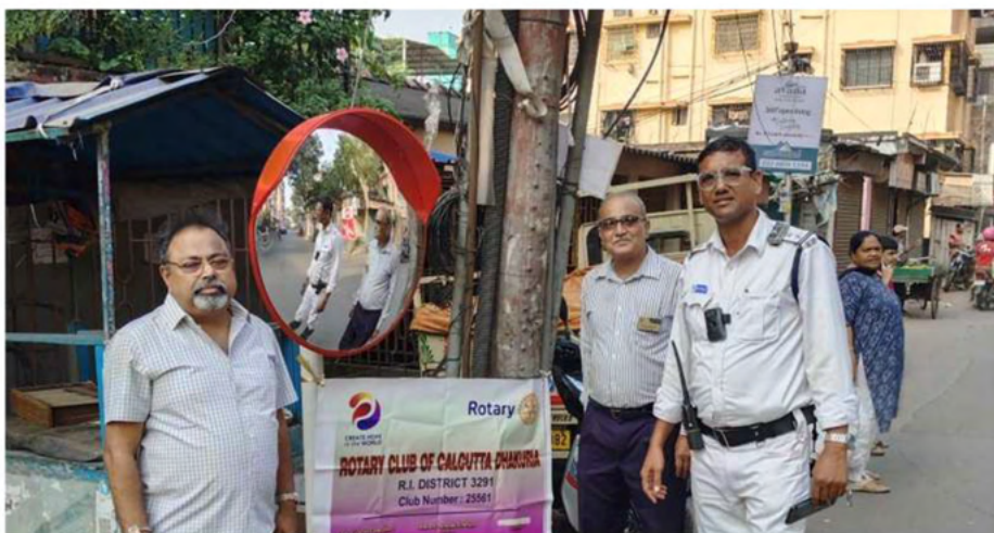
Installation of Convex Mirror at Karunamoyee Ghat Road Junction on 11th November 2023
